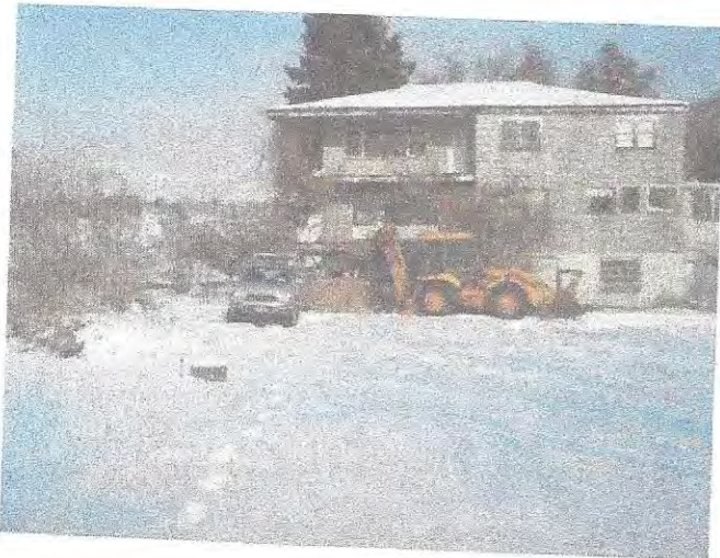
#3 View north showing back of existing home. (Backhoe at Test Pit TP-2)
